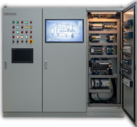
Bio Gas Plant Control Panel
